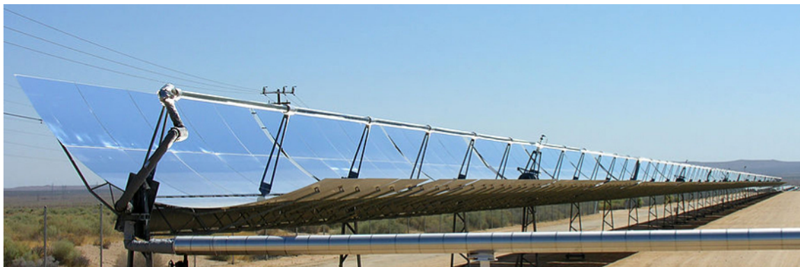
Figure 31.11 Parabolic trough collectors are used to generate electricity in southern California. (credit: “kjkolb”/Wikimedia Commons)
