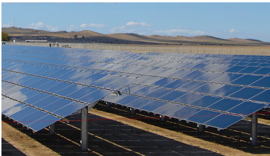
Figure 10.20 Solar cell arrays found in a sunny area converting the solar energy into stored electrical energy. (credit: modification of work by Sarah Swenty, U.S. Fish and Wildlife Service)
